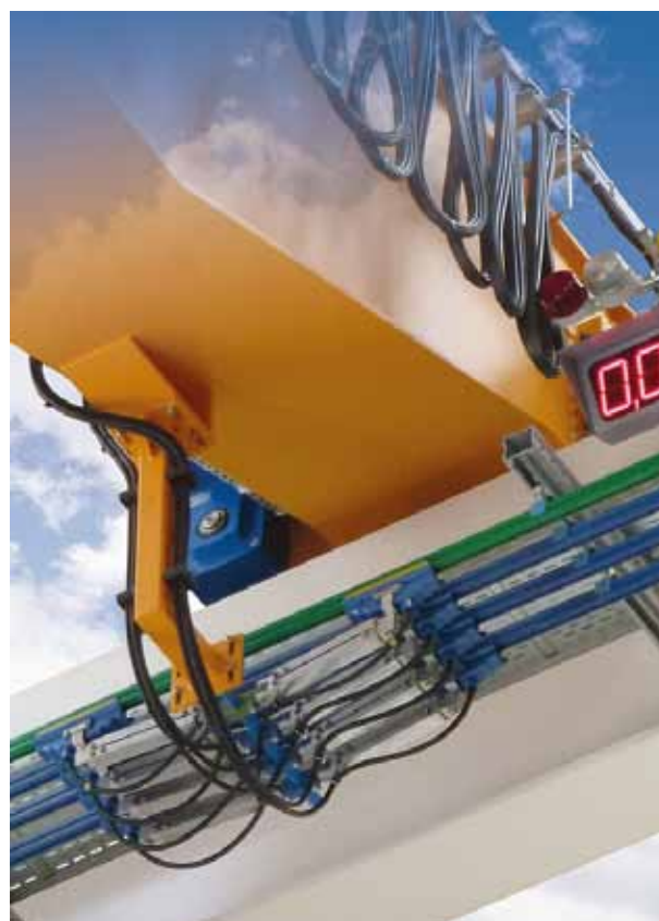
SICL40 system, overhead crane
