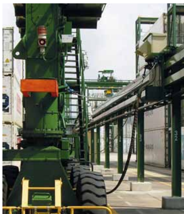
Plug-In/Plug-Out system in RTG operation
